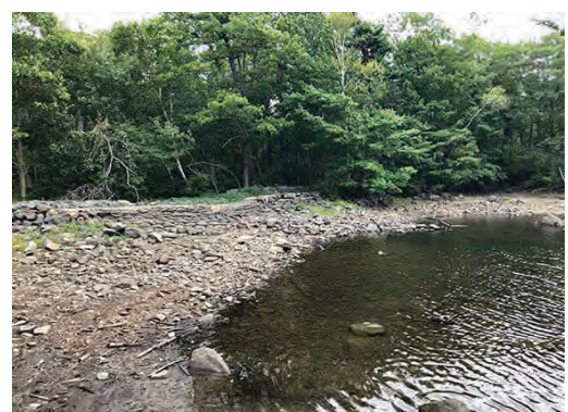
Despite dam being high and dry, as seen here on Sept 10, 2020, water is still flowing out underneath and down the stream on back side
