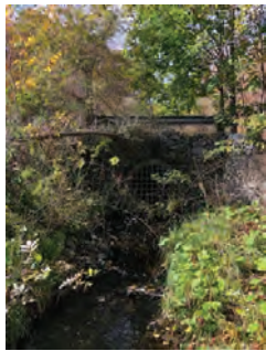
d. Start of Governor's Brook, large pipe in woods, Oct 2
